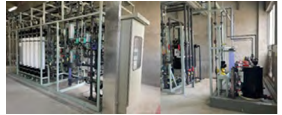
Cooling Tower Blow-down Recovery system
