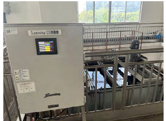
Automatic control system for water treatment chemicals
