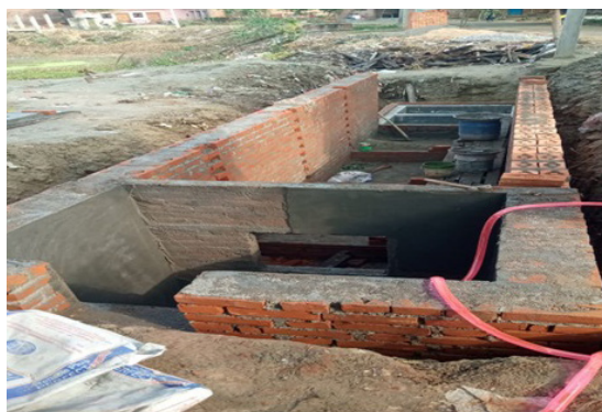
Wastewater treatment system in Uttar Pradesh, India under construction (Courtesy of WaterAid/Archana Pandey)
